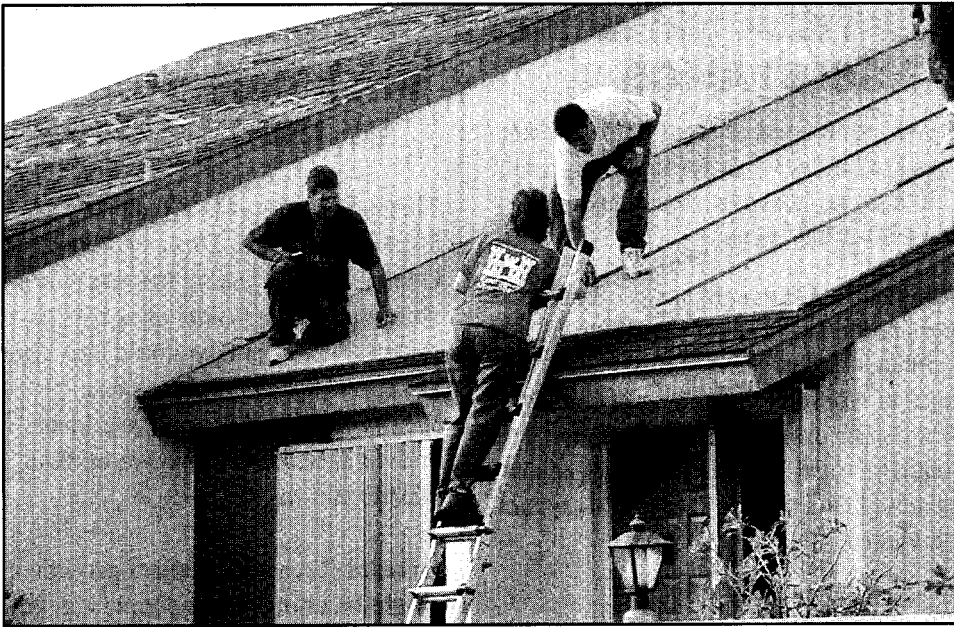
U.S. Army Corps of Engineers staff works with roofers to install a temporary roof as part of the Blue Roof program funded by FEMA. Photo by Dasha Castillo
